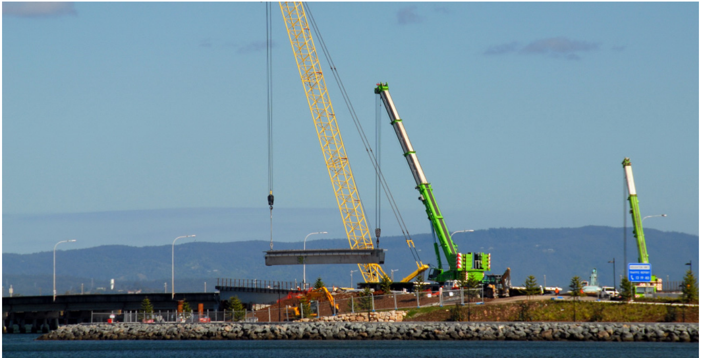
ABOVE: A 35 METRE-LONG, 80-TONNE PRE-CAST CONCRETE GIRDER IS LIFTED INTO POSITION AS WORK CONTINUES ON THE 78 TH SPAN OF THE NEW TED SMOUT MEMORIAL BRIDGE AT CLONTARF POINT. BUILDING THIS SECTION OF THE BRIDGE WILL ASSIST WITH THE CONSTRUCTION OF THE HOUGHTON HIGHWAY'S NEW NORTHERN APPROACH ROADS.
