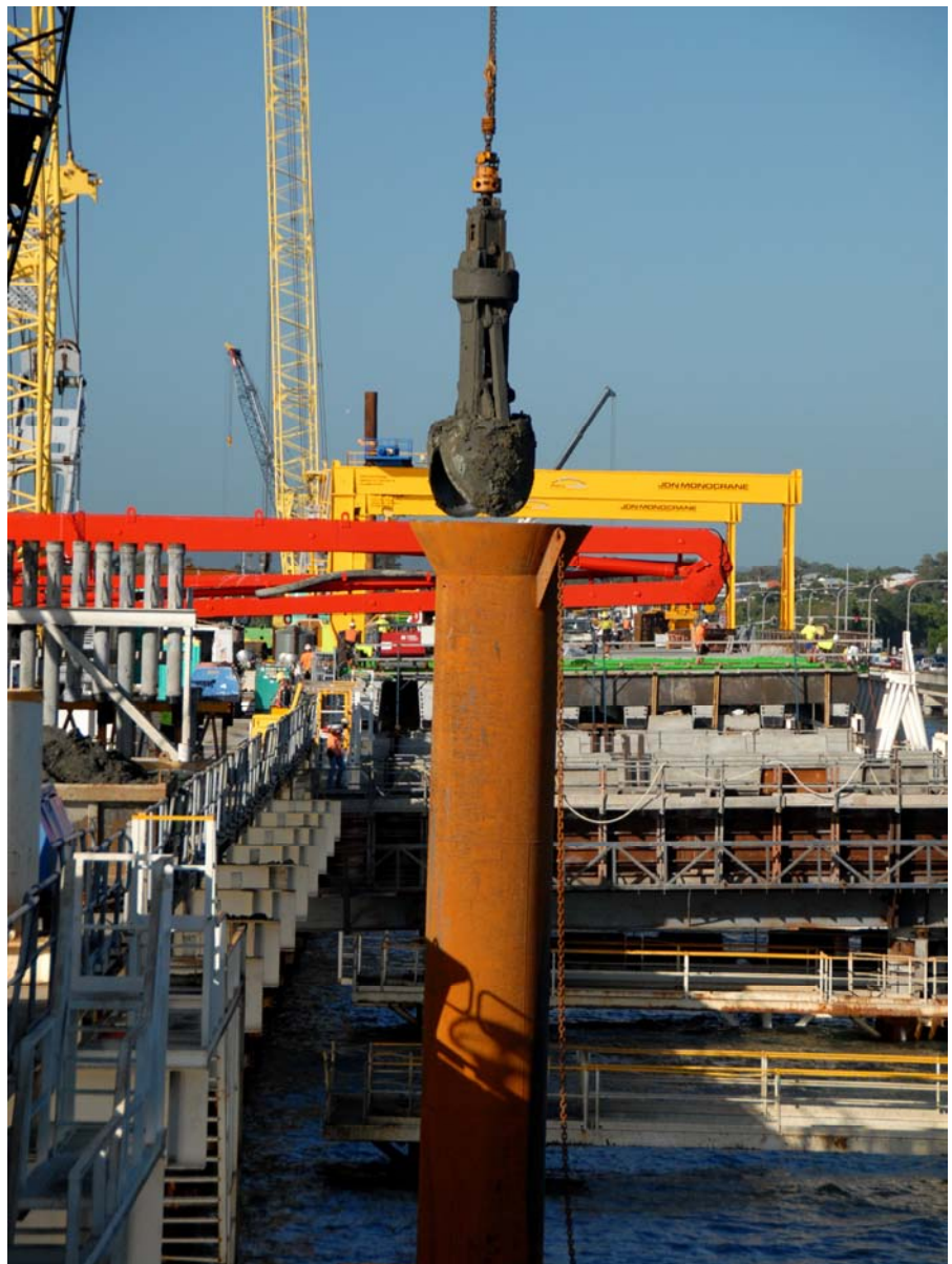
ABOVE: A GRAB-BUCKET REMOVES SEDIMENT FROM THE CORE OF A STEEL BRIDGE PILE SLEEVE THAT HAS BEEN DRIVEN INTO THE BRAMBLE BAY SEABED. THE CORE OF THE SLEEVE WILL BE EXCAVATED, FITTED WITH STEEL REINFORCING, THEN POURED FULL OF CONCRETE.
