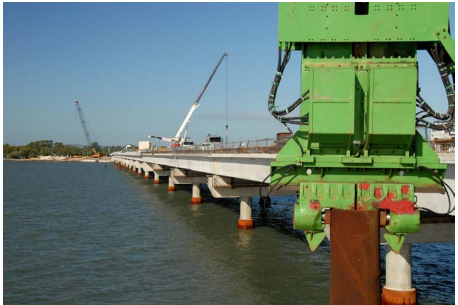
ABOVE: A STEEL PILE FROM THE FALSEWORK CONSTRUCTION PLATFORM BESIDE THE NEW HOUGHTON HIGHWAY BRIDGE IS REMOVED FROM THE SEABED. THE BACK END OF THE PLATFORM IS CONTINUALLY PULLED UP AND LEAPFROGGED TO THE FRONT OF THE STRUCTURE AS THE BRIDGEWORKS ADVANCE NORTH ACROSS BRAMBLE BAY.
