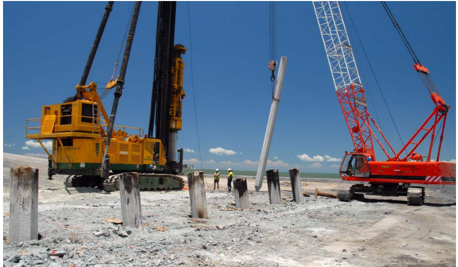
ABOVE: INSTALLATION OF PILES FOR THE NORTHERN ABUTMENT OF THE NEW HOUGHTON HIGHWAY BRIDGE AT CLONTARF POINT.
