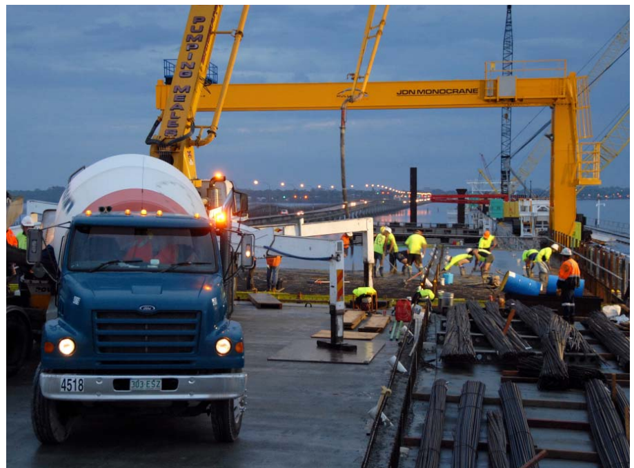
ABOVE: A SPAN OF CONCRETE ROAD DECK BEING POURED ON THE NEW HOUGHTON HIGHWAY BRIDGE.
