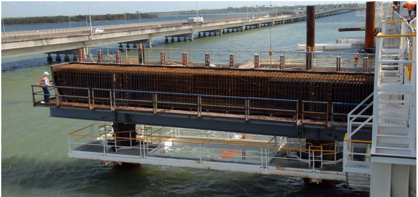
ABOVE: REINFORCED FORMWORK FOR ONE OF THE HOUGHTON HIGHWAY BRIDGE SUPPORT PIERS IS PREPARED FOR FILLING WITH CONCRETE.
