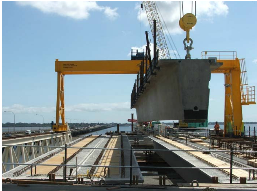
ABOVE: YELLOW GANTRY CRANES LIFT AN 80-TONNE, 35M-LONG CONCRETE GIRDER INTO POSITION OVER THE SECOND SPAN OF THE NEW HOUGHTON HIGHWAY BRIDGE.
