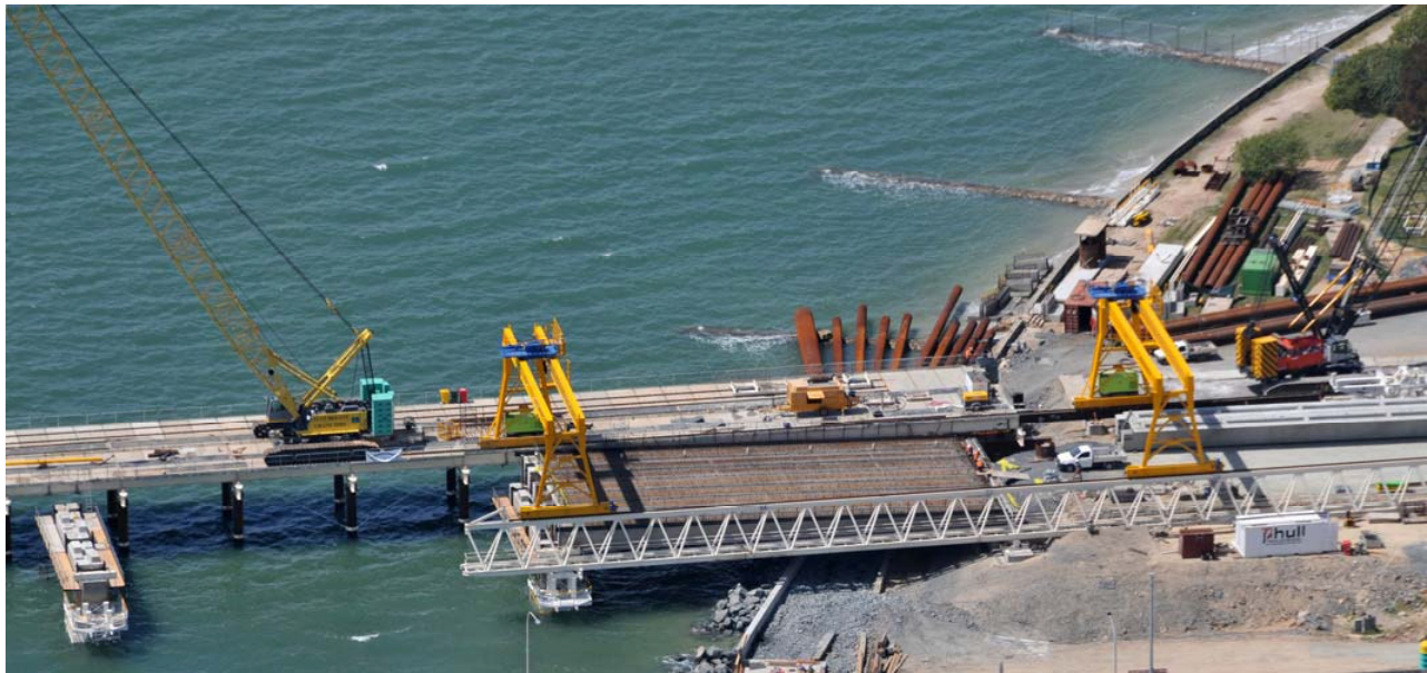
ABOVE: THE FIRST SPAN OF THE NEW HOUGHTON HIGHWAY BRIDGE (FOREGROUND), READY FOR ITS CONCRETE DECK TO BE POURED.
