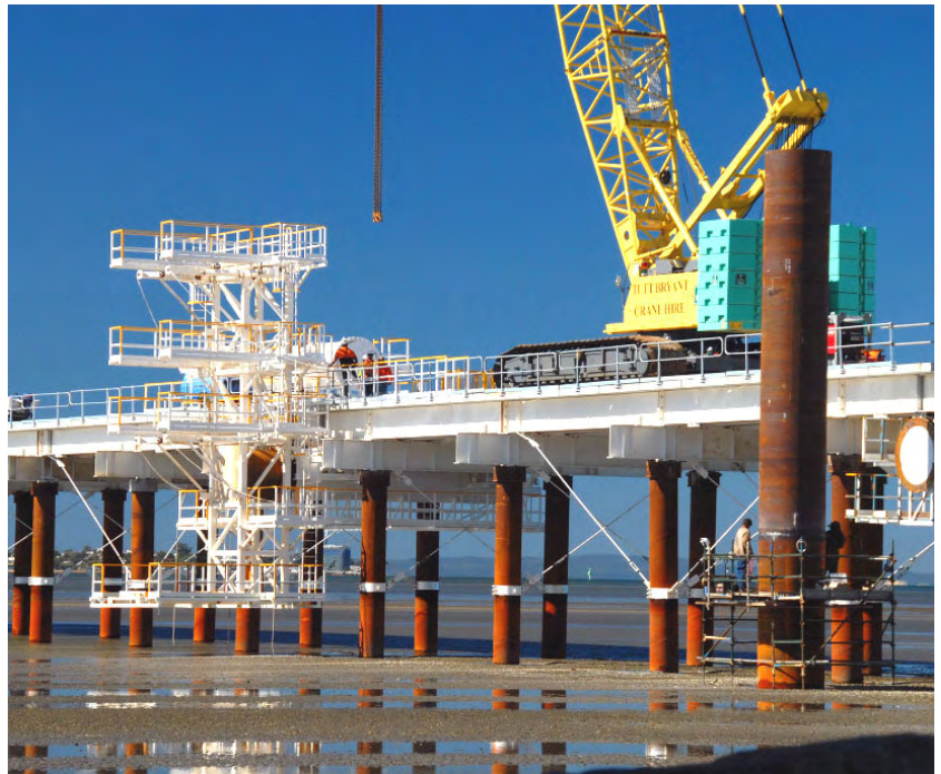
ABOVE: CONSTRUCTION OF THE FIRST SPAN OF THE NEW HOUGHTON HIGHWAY BRIDGE UNDERWAY IN BRAMBLE BAY
