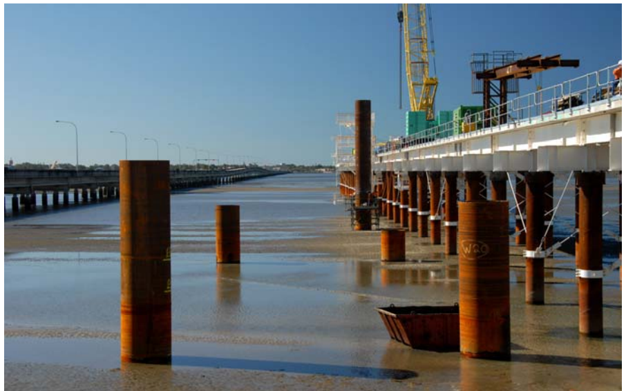
ABOVE: THE FIRST FOUNDATION PILES OF THE NEW HOUGHTON HIGHWAY BRIDGE, INSTALLED IN BRAMBLE BAY IN JULY 2008. THE FALSEWORK BRIDGE IS TO THE RIGHT.
