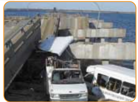
Impacts of Hurricane Katrina on bridges in the United States
