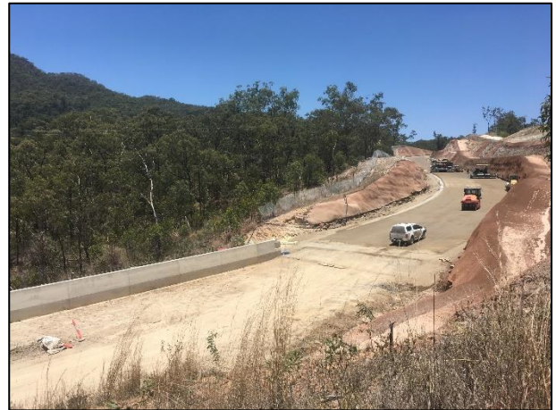
Plate 2: Construction traffic/ hazards
