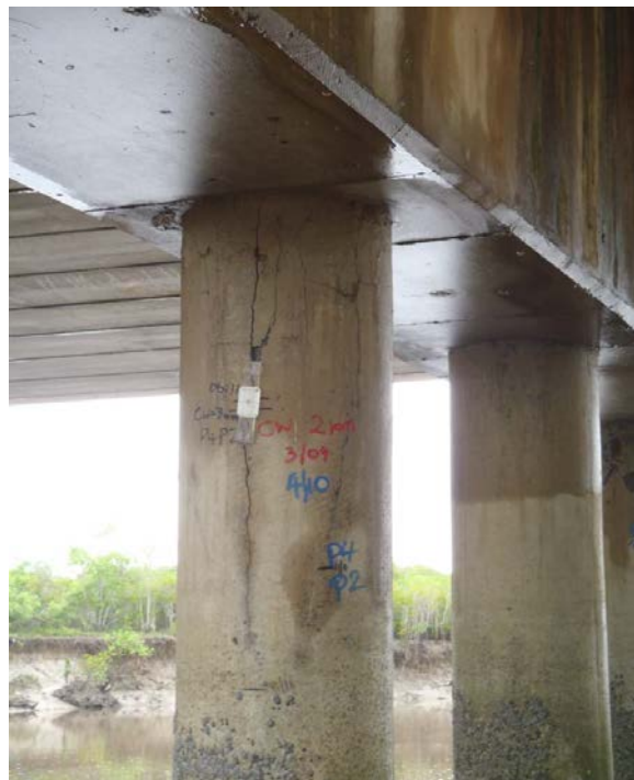
Figure 5.1.2-7: Cracking in piles with crack monitoring in place
