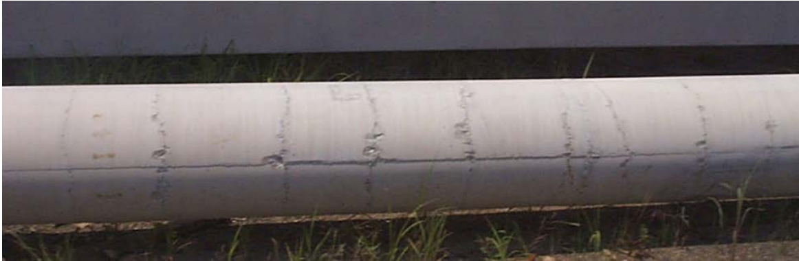
Figure 5.1.2-2: Cracking at the head of a hollow spun pile
