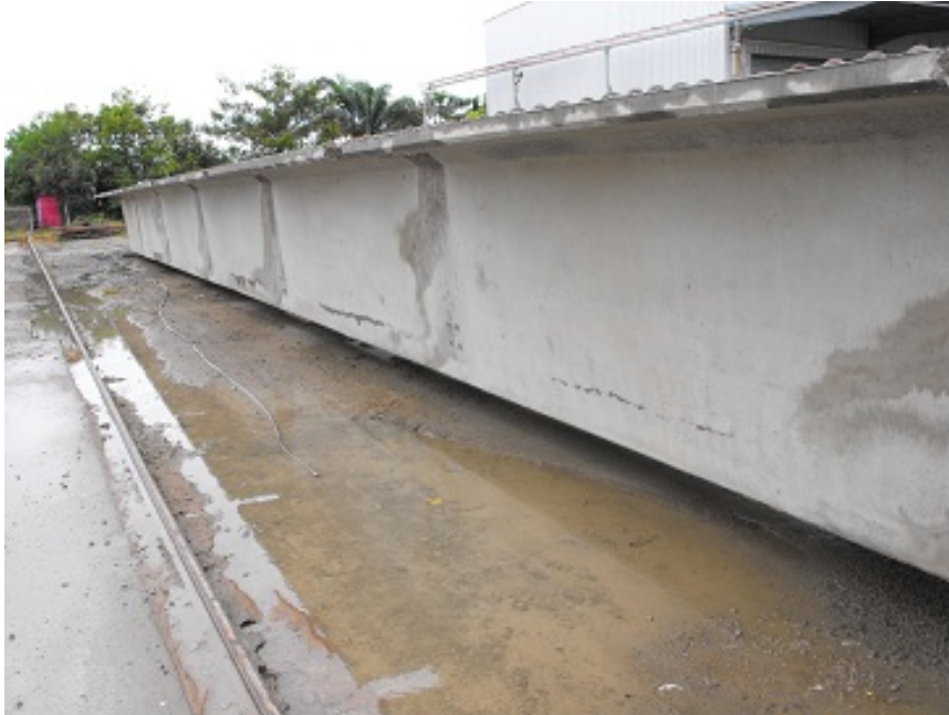
Figure 15 – Poor quality concrete due to heat of hydration
