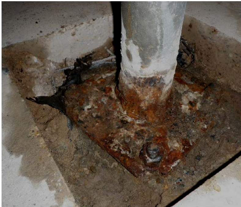
Figure 8.2- 3 – Corrosion of post buried in concrete where water has seeped in
