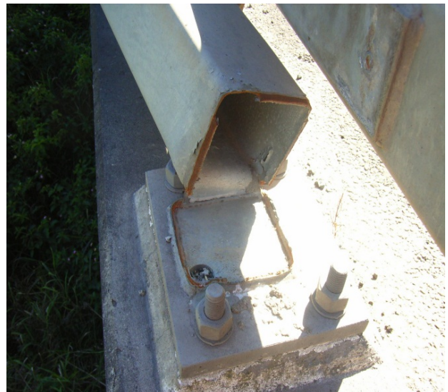
Figure 9.4-2 - Posts fillet welded – not butt welded as required on drawings
