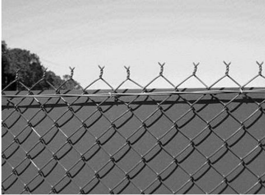
Figure 6.11.2 Incorrectly installed fauna exclusion fencing. For correct installation details refer to Main Roads Standard Drawing 1603.
