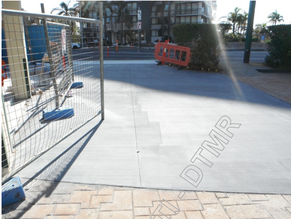
Figure 3 – D’Arcy Arms Northern Driveway
