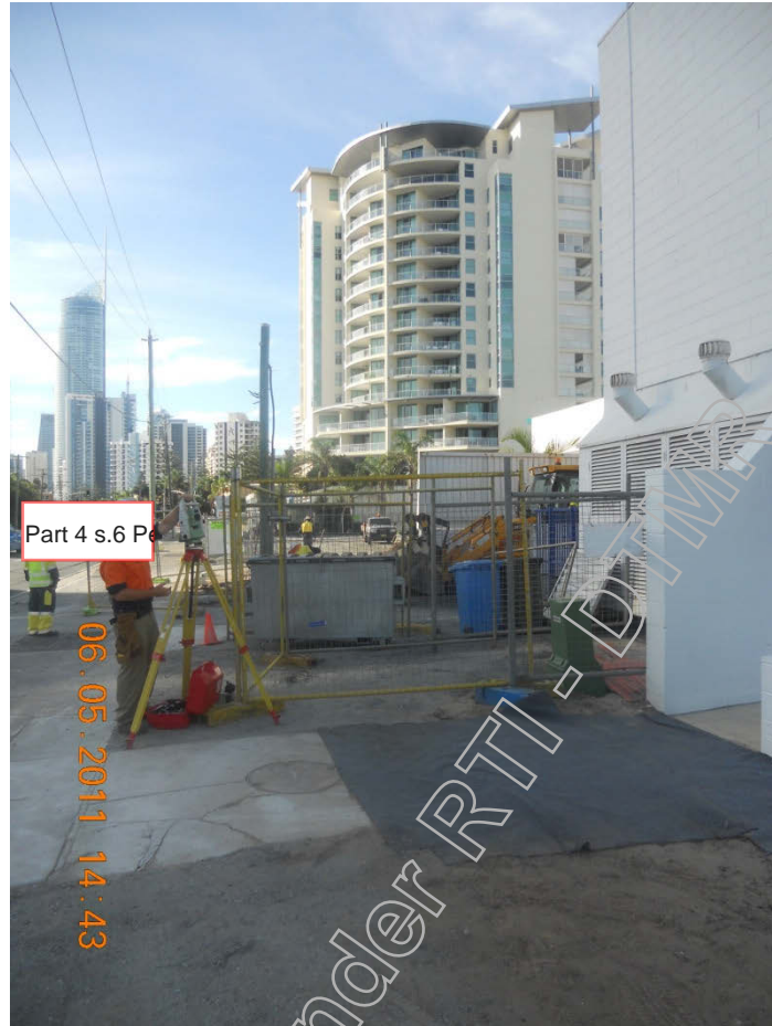
Telstra Pit (Manhole 89) location after removal of Energex padmount transformer (Critical path work)
