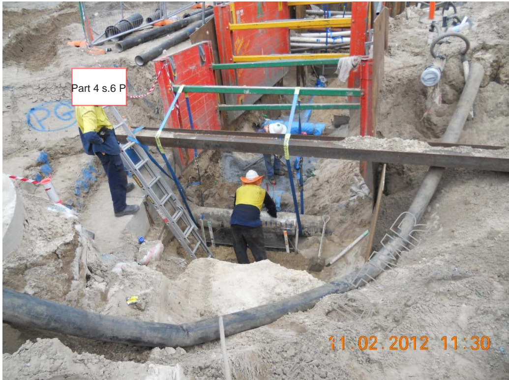
Figure 3: Thrust Block Pour of the WD2 WM for the Scour Connection at Rosewood Avenue
