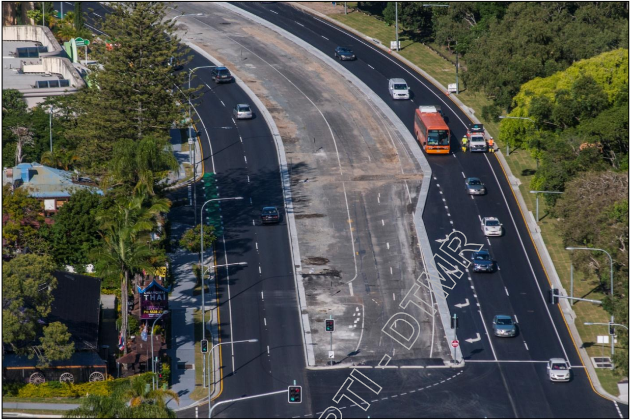
Figure 2: Aerial View of the new Pavement and Line Marking Looking South from St. Kilda Av
