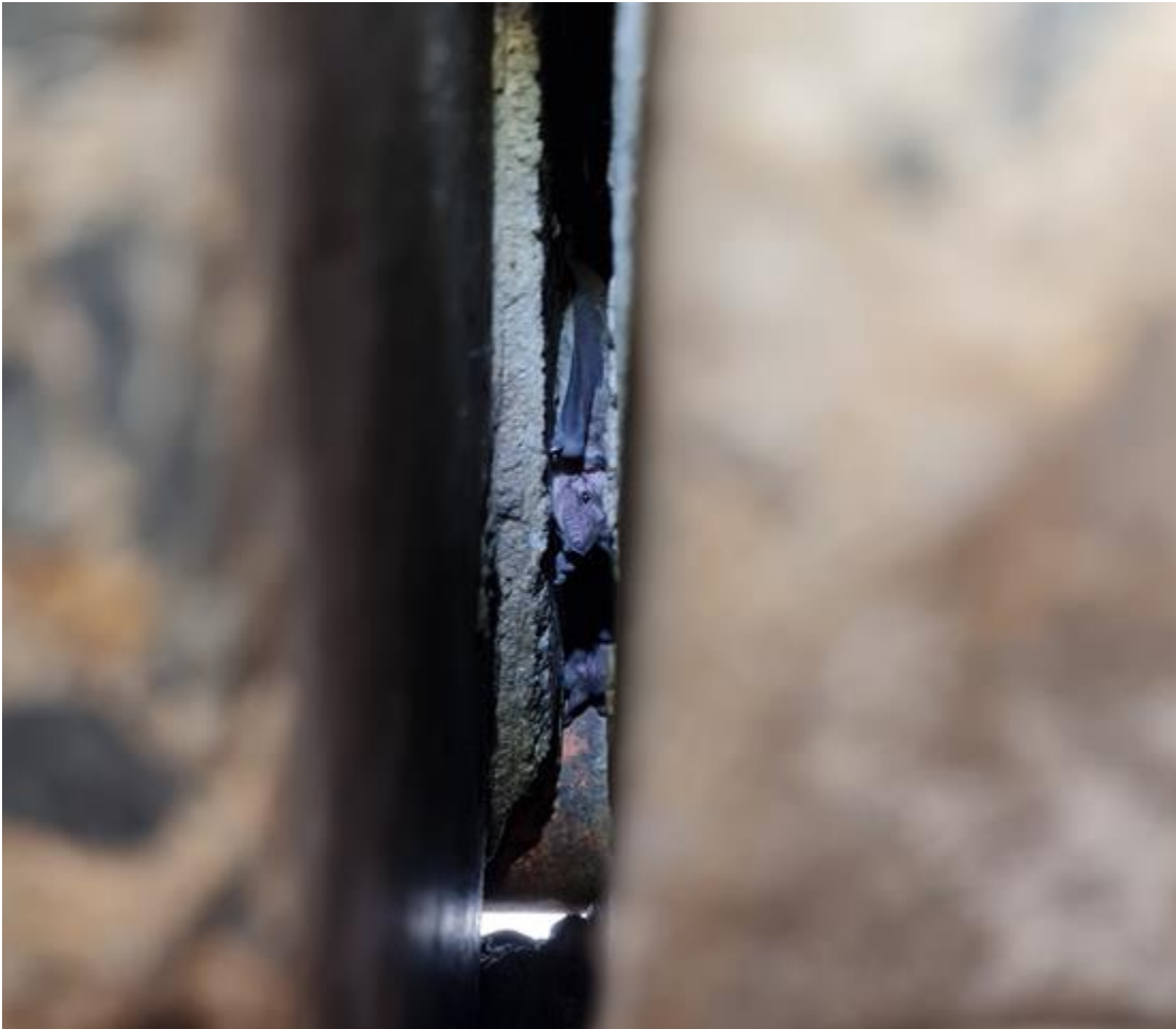
Eastern freetail bat ( Ozimops ridei ) in the expansion joint at Lockyer Creek Bridge
